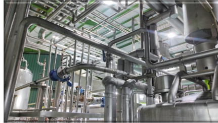
Figure 16: Joints Between Stainless Steel Pipe and Fittings Shall Comply with Sections 605.22.1 Through 605.22.3 of the IPC.
