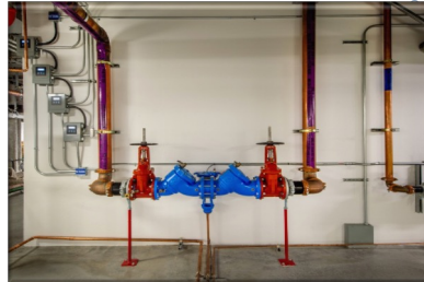
Figure 18: Backflow Preventer System
