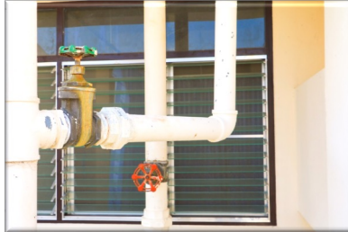
Figure 13: Piping Should Not Interfere with Normal Operation of Windows, Doors or Other Means of Egress
