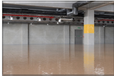
Figure 3: Plumbing systems installed in flood hazard areas shall be in accordance with IBC
