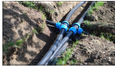
Figure 15: Water Service Pipes Shall Not be Less Than \frac{3}{4} Inch in Diameter
