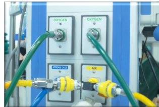
Figure 5: Medical Gas System
