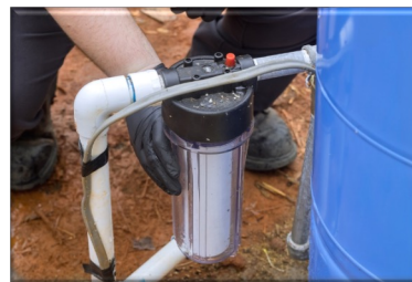
Figure 9: Filtration is required when using Non-Potable Water for Water Closet and Urinal Flushing Applications
